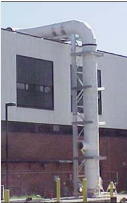
Odor Control Duct Systems for Water Treatment
