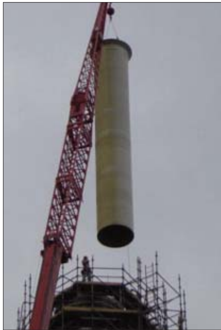
Stack Liner, 6' Diameter x 40' Section of 200' Stack
