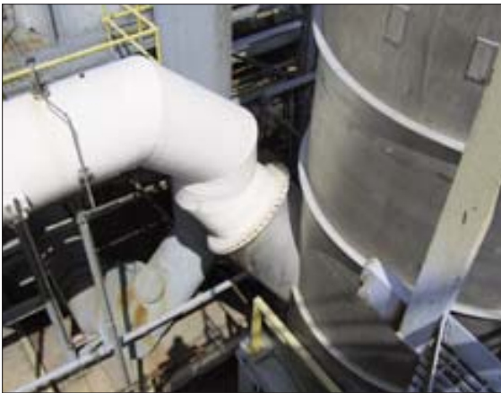
Industrial, Corrosion Resistant Duct
